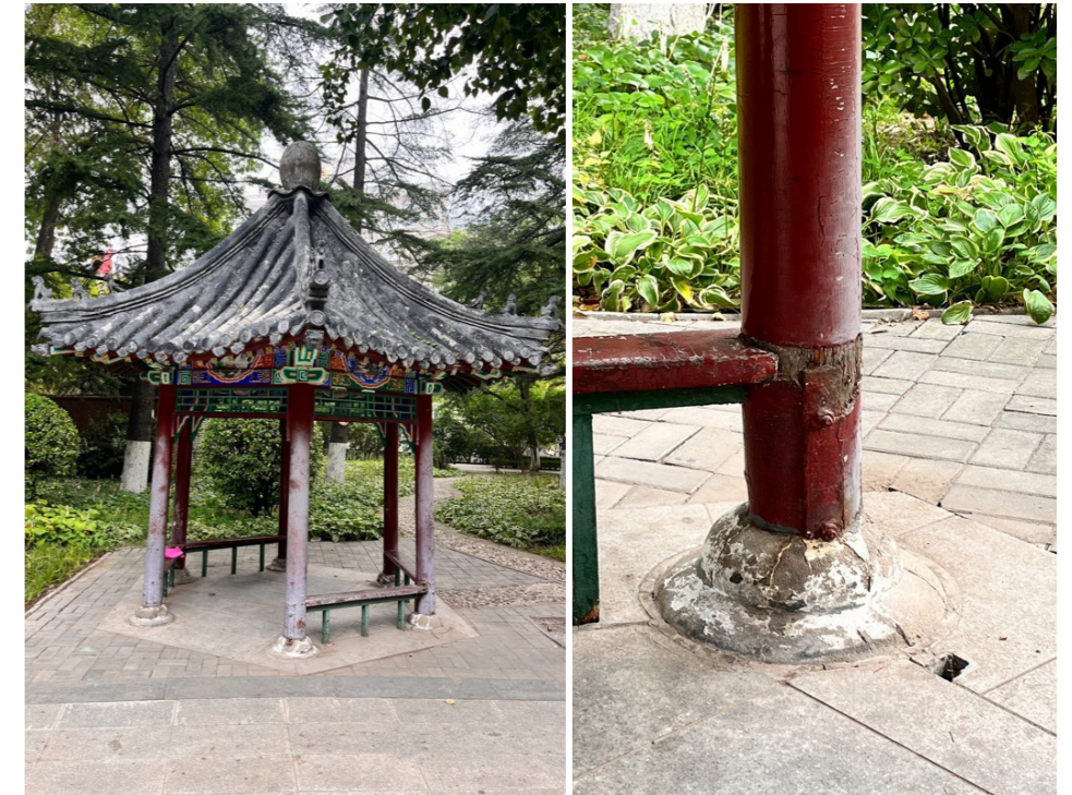
Figure 5-2. Historic elements in disrepair in Jiefang North Park Source: Yue LU in 2023
